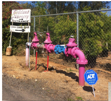
Recycled water program
