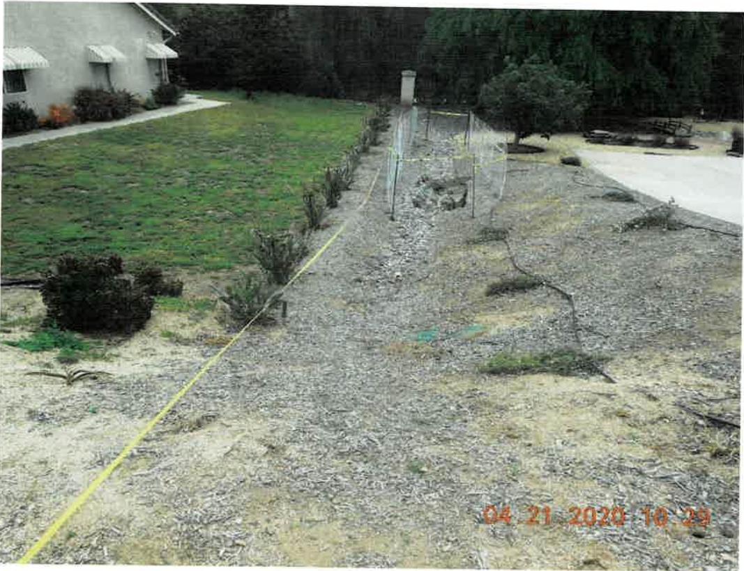
04-21-2020 Photos of expanding hole after putting up fence to keep people and animals out.
