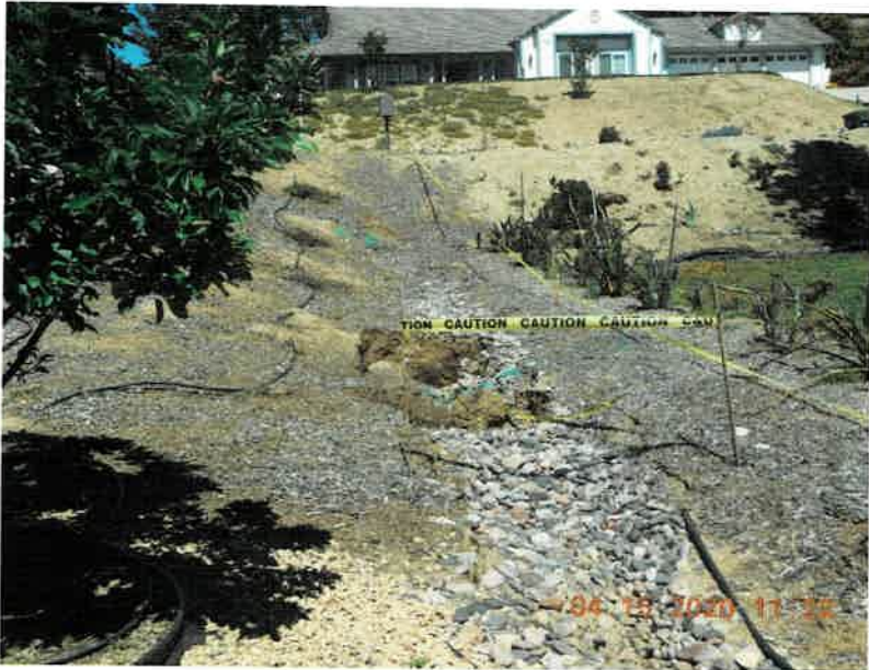
Photo from below major damage from below looking up towards Palomares Road, at about 50 feet from Palomares Road
