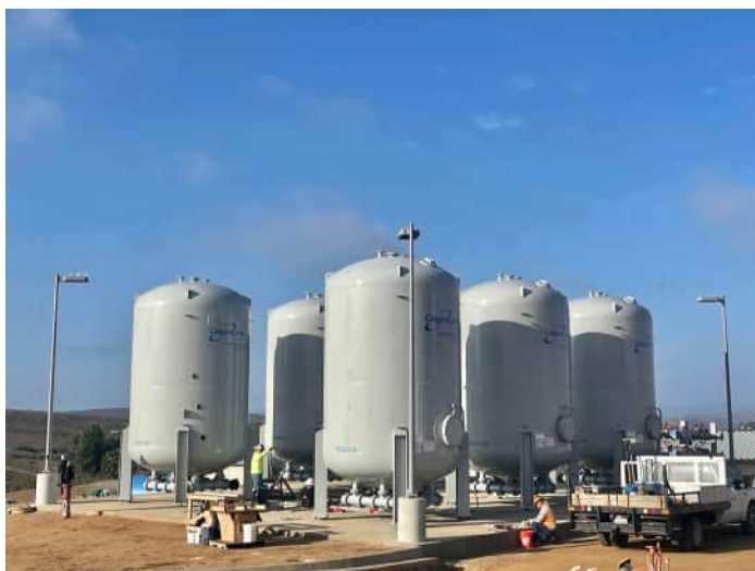
Santa Margarita Groundwater Treatment Plant (SMGTP)
