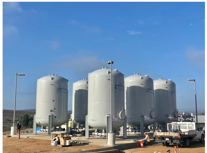
Santa Margarita Groundwater Treatment Plant (SMGTP)
